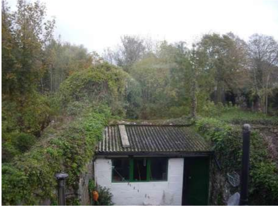
Fig 19 Image taken from rear of New Street showing the town wall between the gardens of 12 and 13 New Street.
