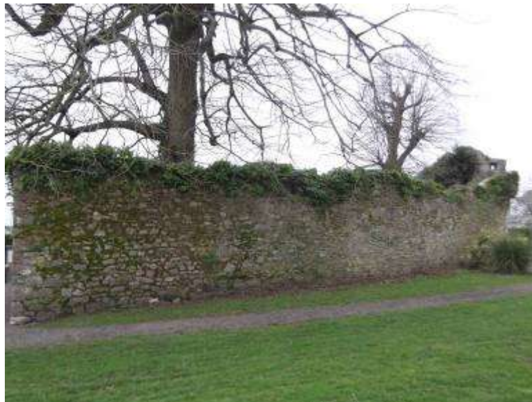
Fig 23 External Face of East Wall, the internal face is not readily accessible as it is located to the rear of the Tennis Clubhouse, note bartizan to the right and location mature tree.
