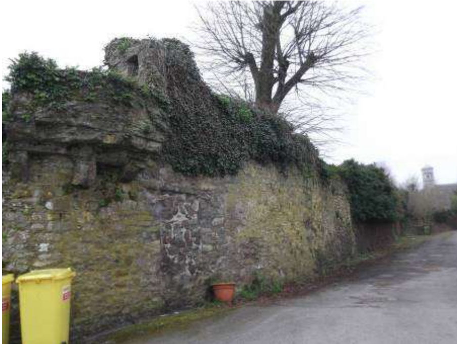
Fig 22 North wall external face. Note blocked up former opening, Bartizan and mature tree.
