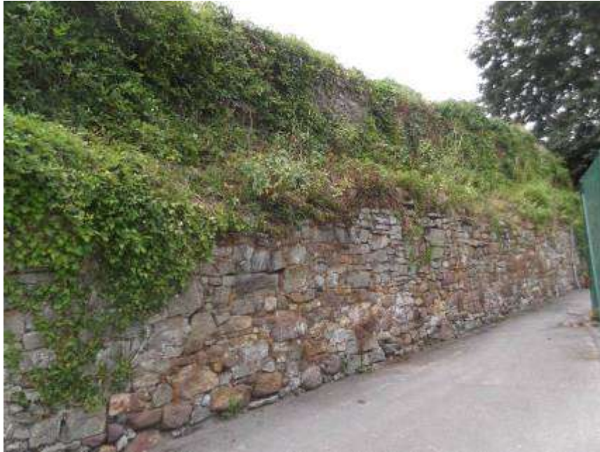
Fig. 11 Internal face of walls at the tennis Courts. No presence of wall walk.
