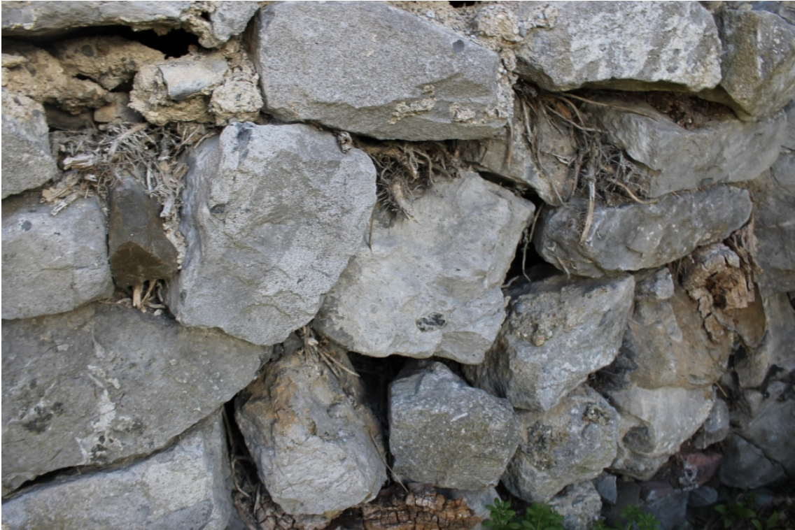
Area 2 – Internal Face – Note Woody Ivy Stems & Open Joints - Taken 24/10/14
