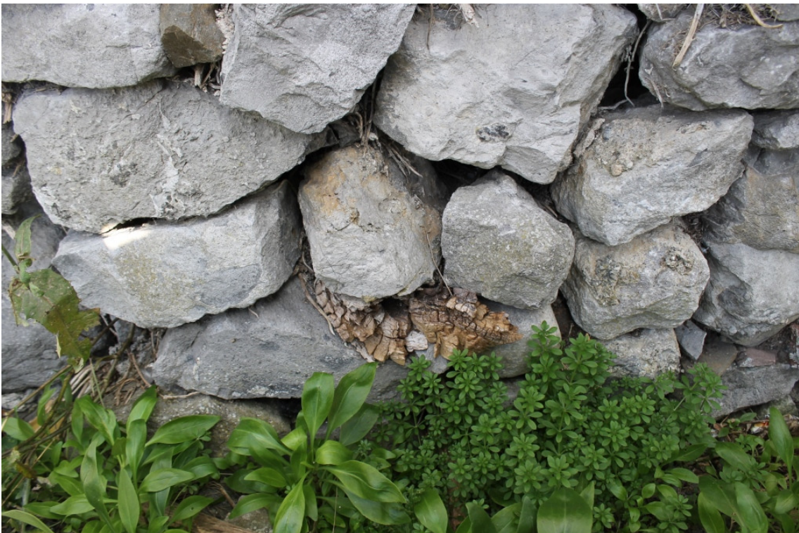
Area 2 – Internal Face – Note Woody Ivy Stem & Open Joints - Taken 24/10/14
