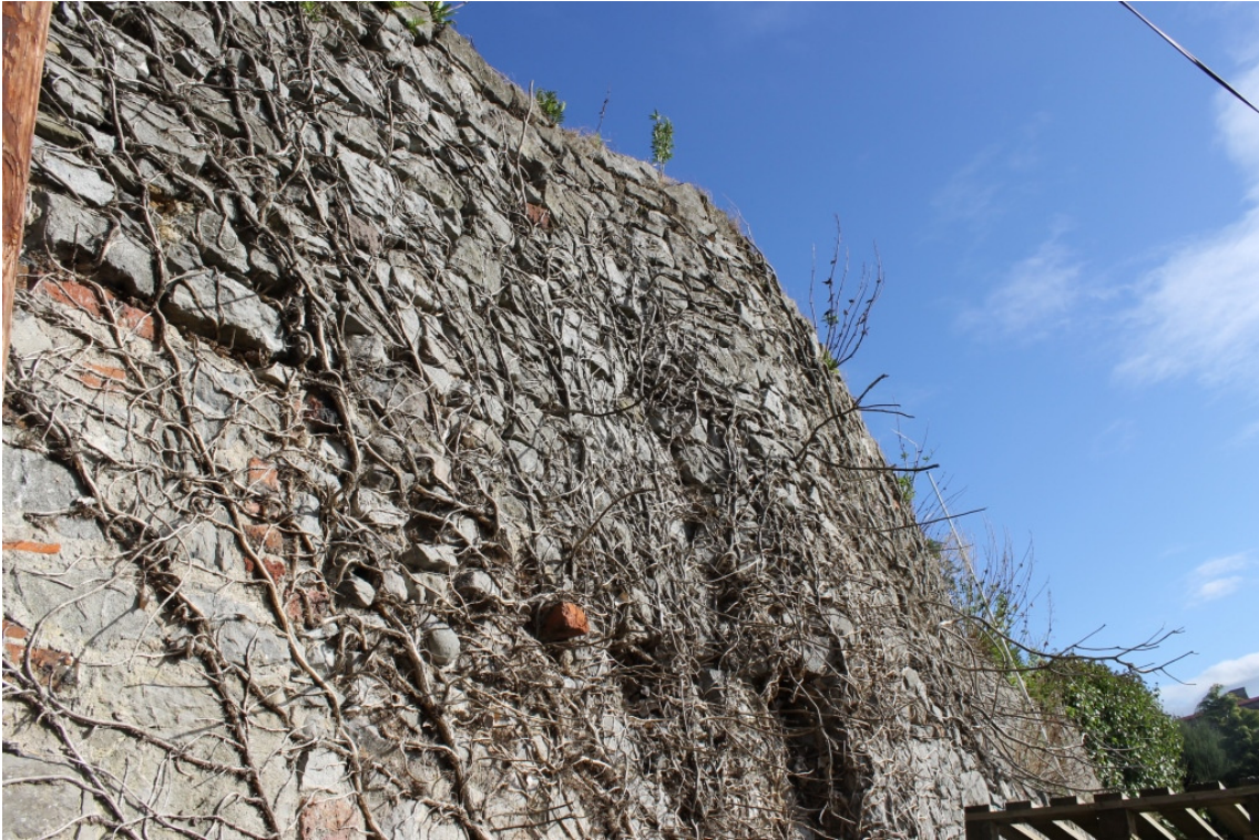
Area 2 – Internal Face – Note Curved Section of Wall and Dead Ivy - Taken 24/10/14
