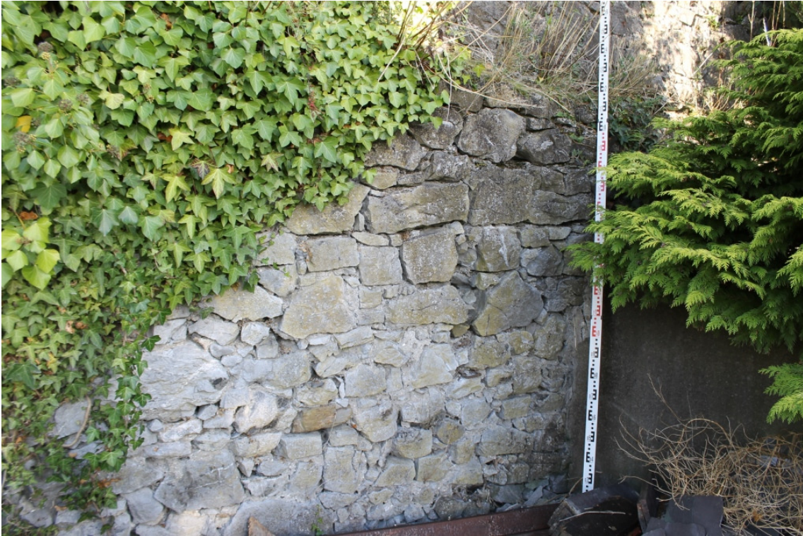
Area 2 – Internal Face – View of Wall to South of Area 2 – Note Open Joints - Taken 24/10/14
