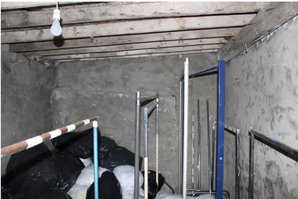
Area 1 - Internal Face – Note Step in Wall & Cement Render – Taken 24/10/14
