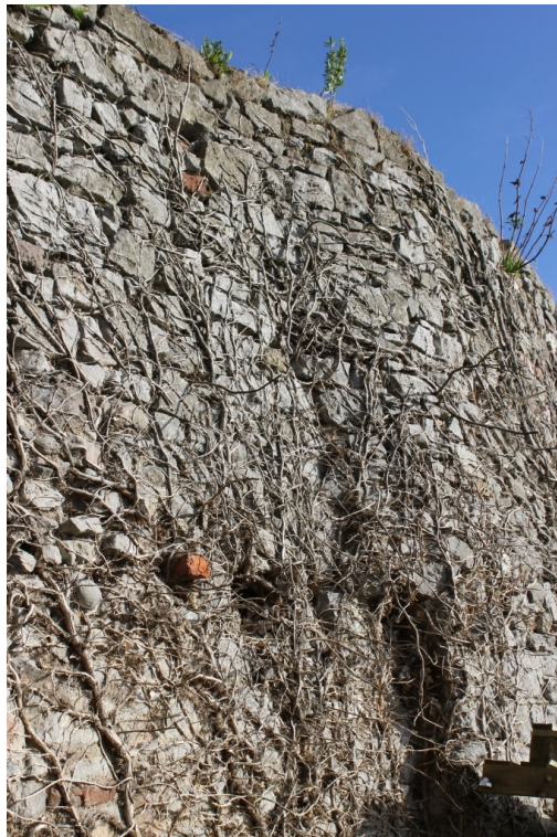
Area 2 – Internal Face – Note Curved Section of Wall and Dead Ivy - Taken 24/10/14
