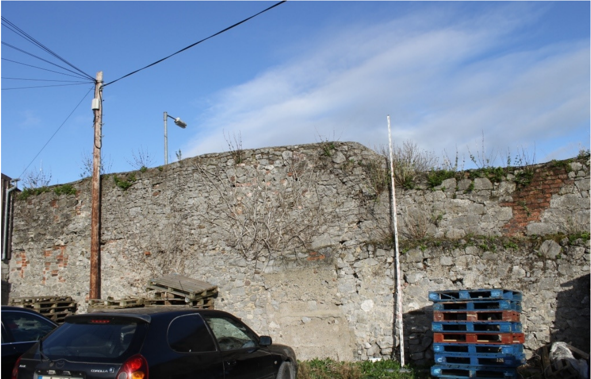
Area 2 – Internal Face – Note Concrete patching to Left of Staff - Taken 24/10/14
