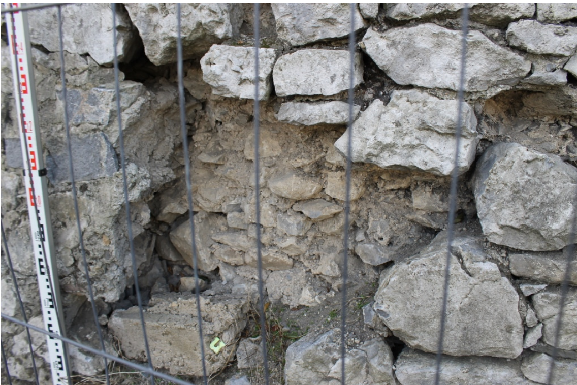
Area 1 – External Face – Note Previous Attempts to Fill Void with Concrete - Taken 24/10/14
