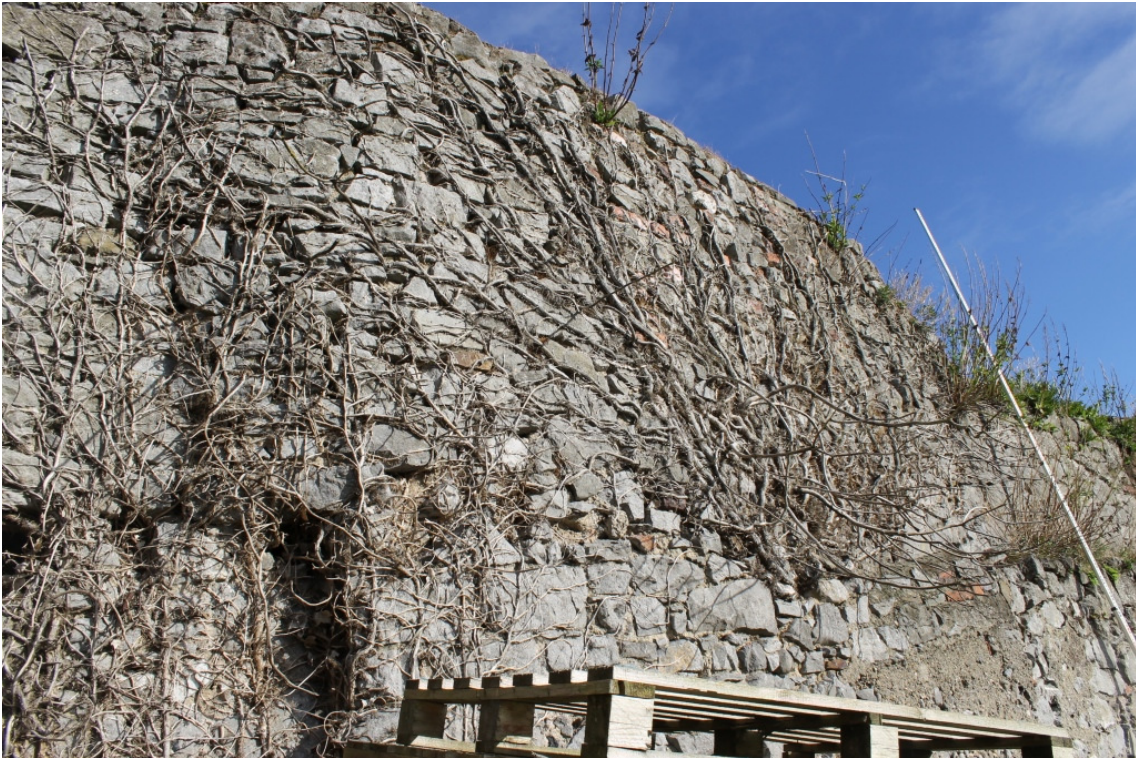
Area 2 – Internal Face – Note Curved Section of Wall and Dead Ivy - Taken 24/10/14
