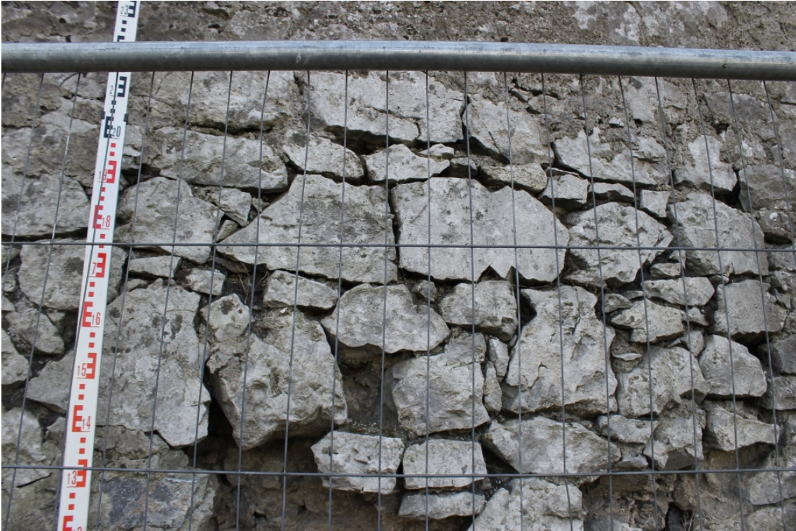
Area 1 – External Face – Note Open Joints Over Void Section - Taken 24/10/14
