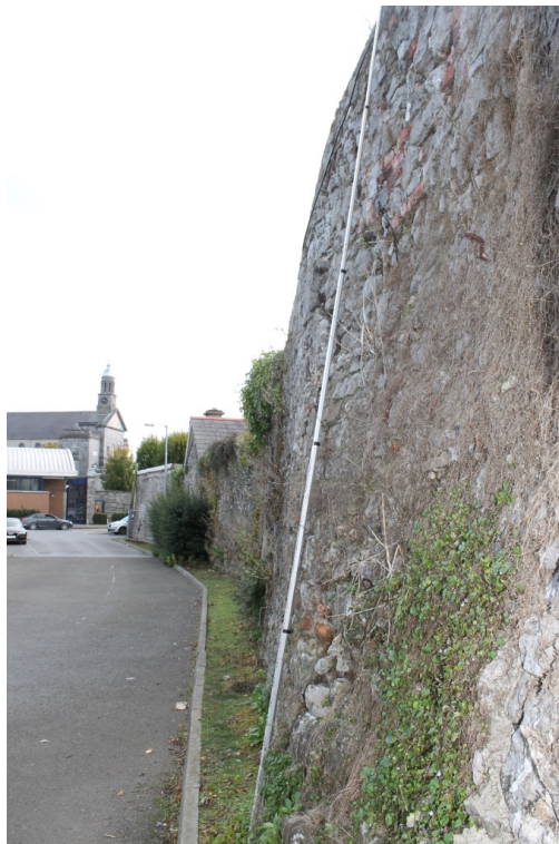
Area 2 – External Face – Note Taper/Lean in Wall – Taken 24/10/14
