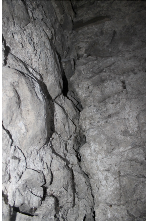
Area 1 – Internal Face – Cracking at Junction with Internal Division Wall - Taken 24/10/14
