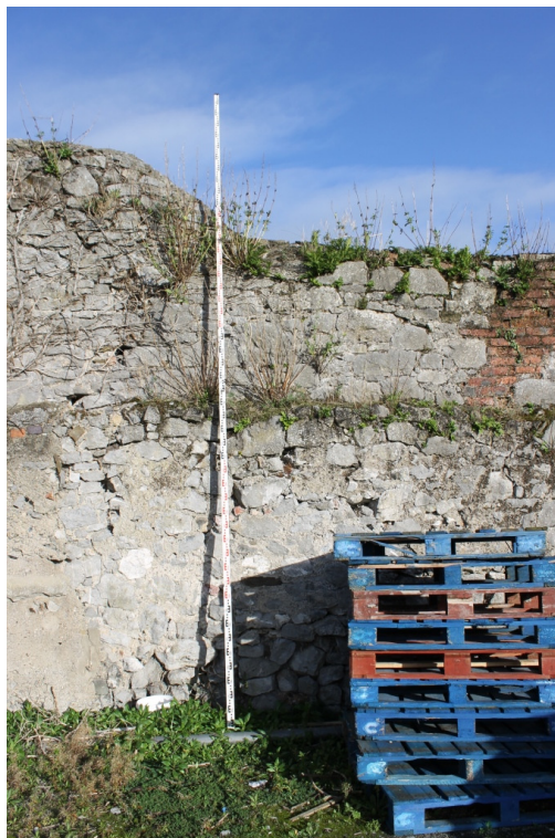
Area 2 – Internal Face – Note Dead Plant Growth Along Step - Taken 24/10/14
