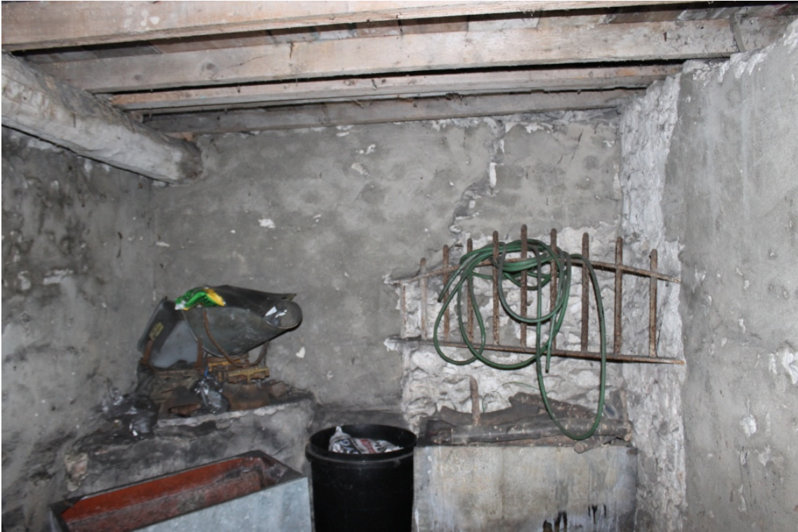
Area 1 - Internal Face – Note Cement Render & Projection in Wall – Taken 24/10/14
