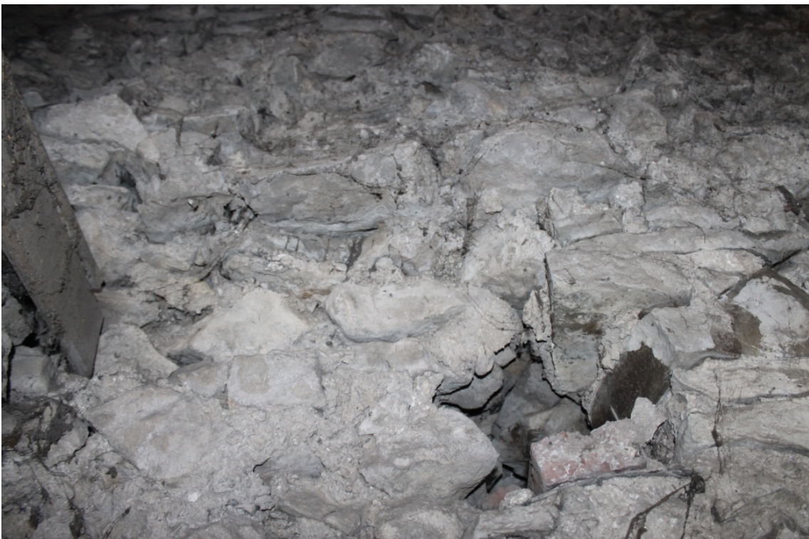
Area 1 – Internal Face – Open Joints and Void in Wall - Taken 24/10/14
