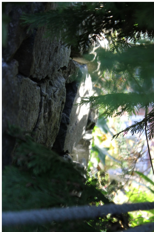
Area 2 – Internal Face – View of Wall in Garden to South of Carpark - Taken 24/10/14
