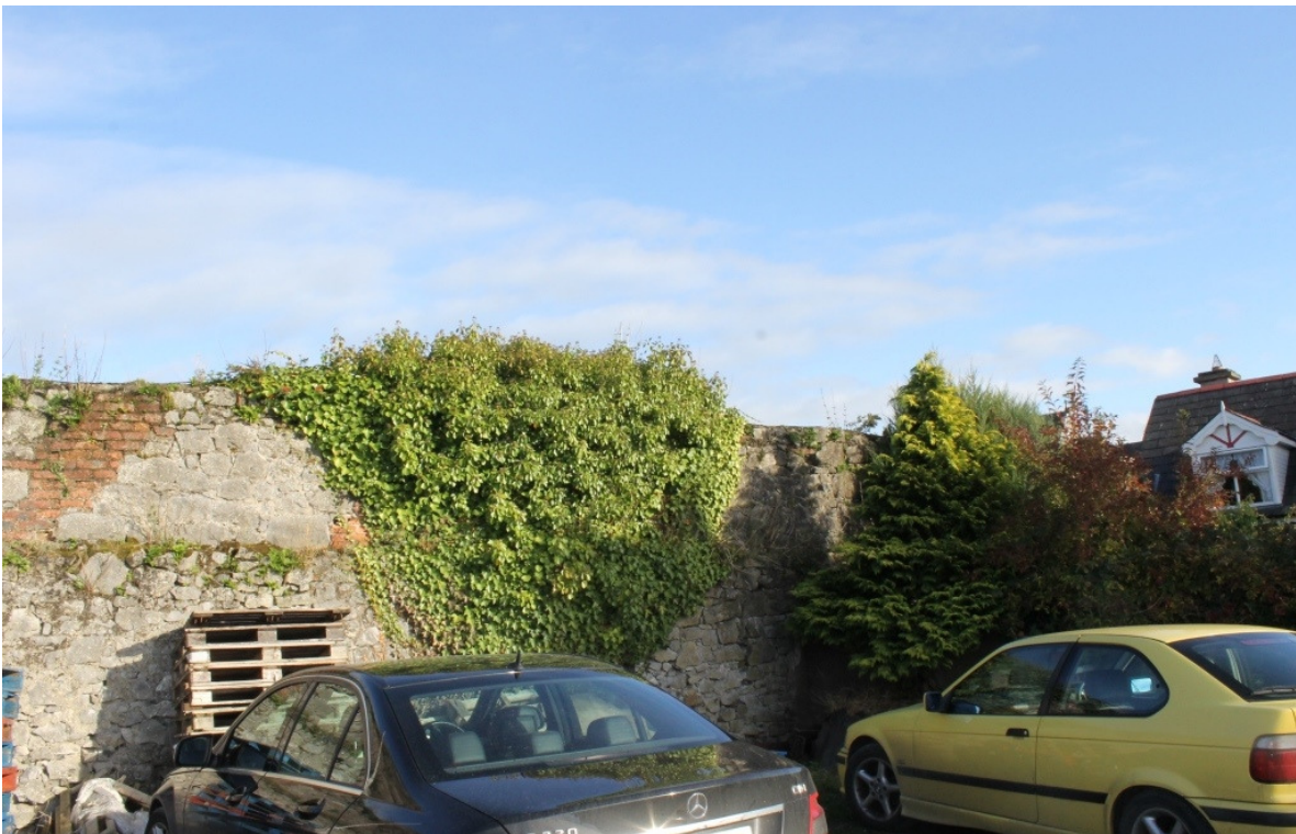
Area 2 – Internal Face – Note Ivy Growth and Proximity of Tree - Taken 24/10/14
