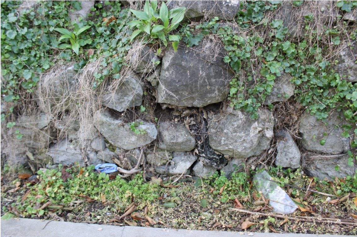
Area 2 – External Face – Note Significant Ivy Stem in Wall – Taken 24/10/14
