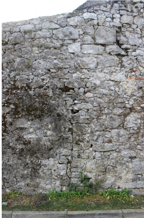
Area 2 – External Face – Note Step in Wall and Possible Previous Opening – Taken 24/10/14
