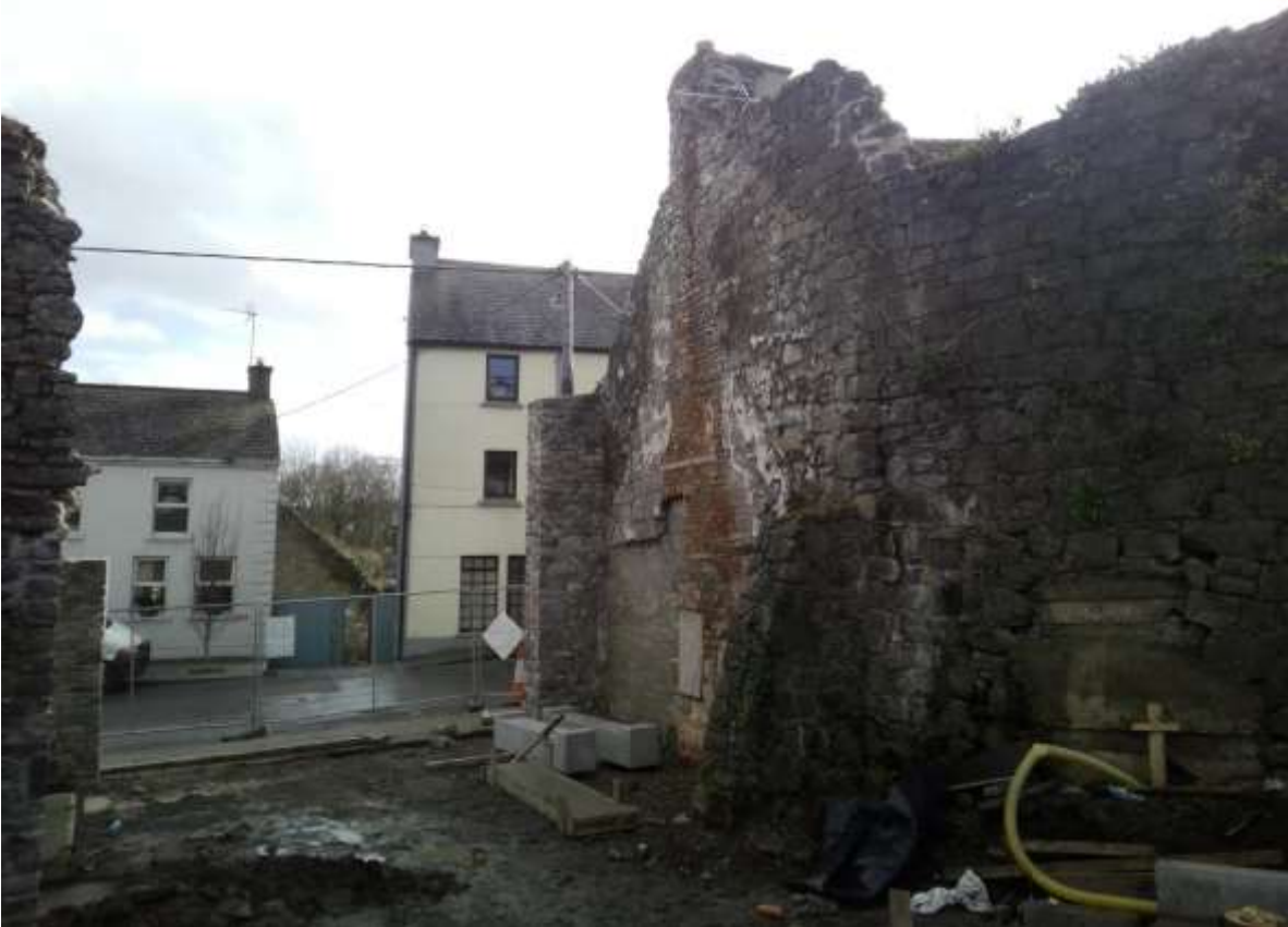
8. Section of wall at entrance to new park from Burke St. The gable wall and upper portion of the town wall have been partly conserved. There is a blockwork infill panel at the base of this wall, which will be finished with a lime harling as part of the proposed works.
