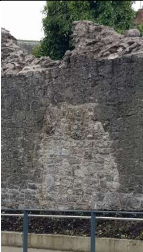
v. Southern part of wall, with reinstated stone rubble infill within earlier opening – 7/11/19
