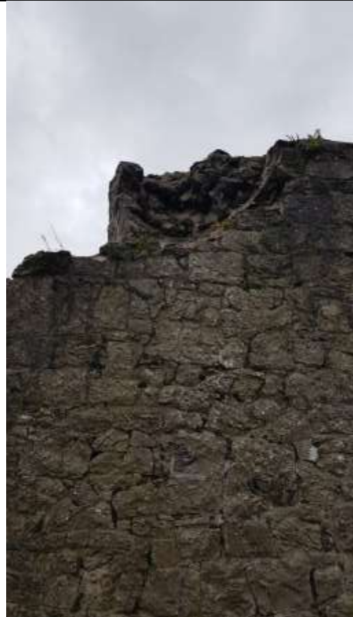
viii. Detail of part of the top of the wall, where the existing stone rubble was consolidated and re-pointed with limecrete to ensure water run-off – 7/11/19
