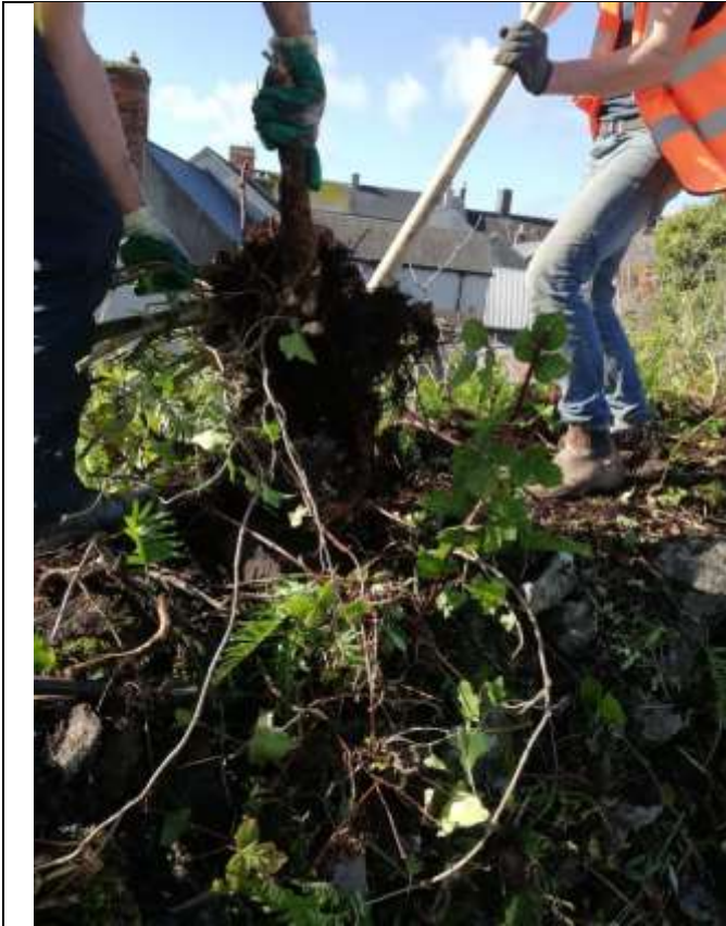
ix. Removal of vegetation from top of wall during works – progress photo October 2019
