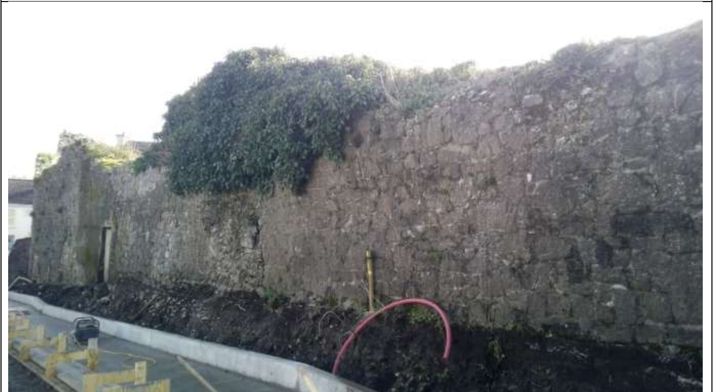
4. Significant ivy growth and vegetation on upper part of wall. This vegetation threatens the fabric of the wall and is to be removed in tandem with the re-pointing and consolidation of the wall.
