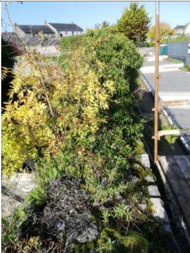
12. Top of wall (looking north), showing extent of vegetation growth within the core of the wall prior to the commencement of work – October 2019
