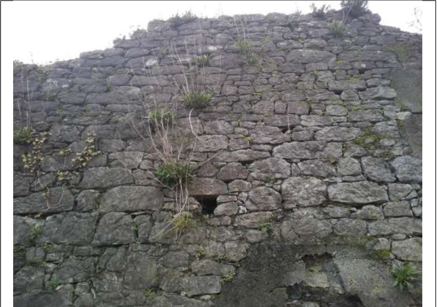
3. Detail of south part of subject wall (close to Burke Street) prior to works. The haunching at the top of the wall has broken down with colonisation by buddleia and ivy. There are loose and unstable stones along the top of the wall.
