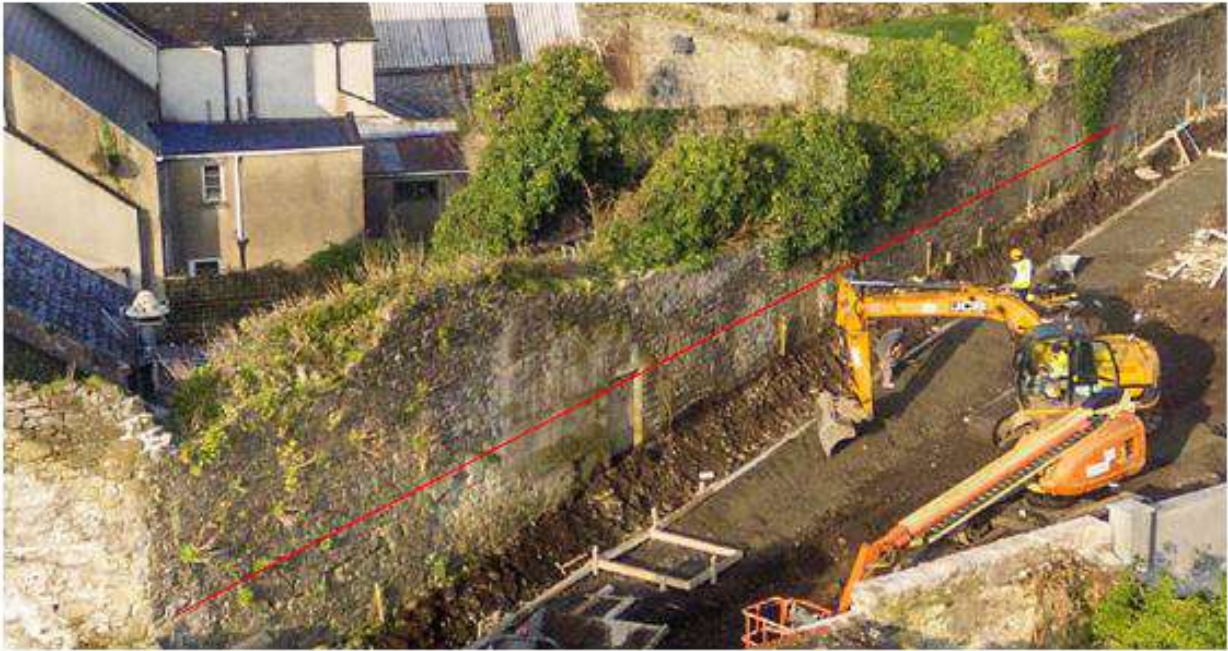
1. Southern part of wall, where the impact of ivy growth on the top of the wall was particularly bad, prior to work
