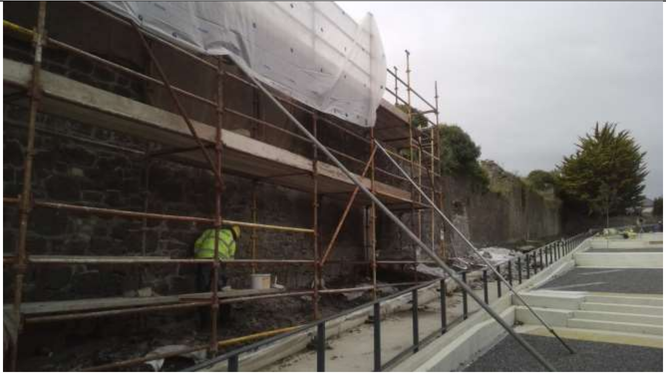
xiii. Progress photograph showing scaffolding in place on southern part of wall, with re-pointing underway – October 2019
