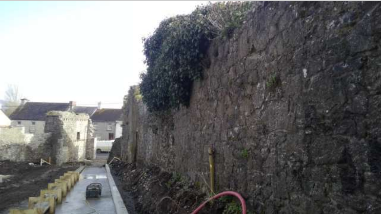
6. General view showing the presentation of the town wall within the new park. The upper part of the wall has been colonised by heavy ivy growth, which has broken down the haunch and threatens the stability of the wall.
