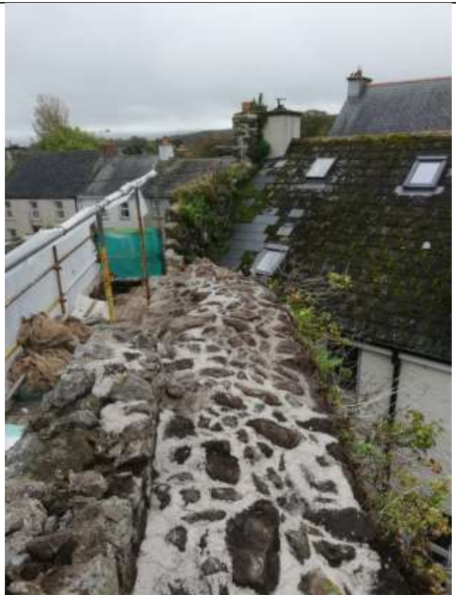
xii. Work in progress, pointing top of wall with limecrete haunch – progress photo October 2019
