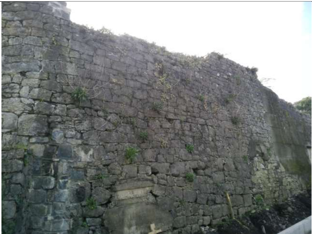
2. This photograph (prior to the works) shows the southern part of the subject wall (northeast face), viewed from within the new park. There are areas of missing mortar, together with gaps and cavities associated with missing stones.
