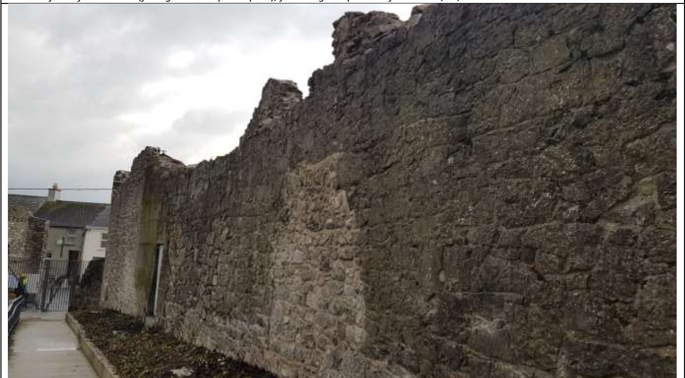
ii. Southern part of wall, with consolidated masonry at top of wall and reinstated stone rubble infill within earlier opening – 7/11/19
