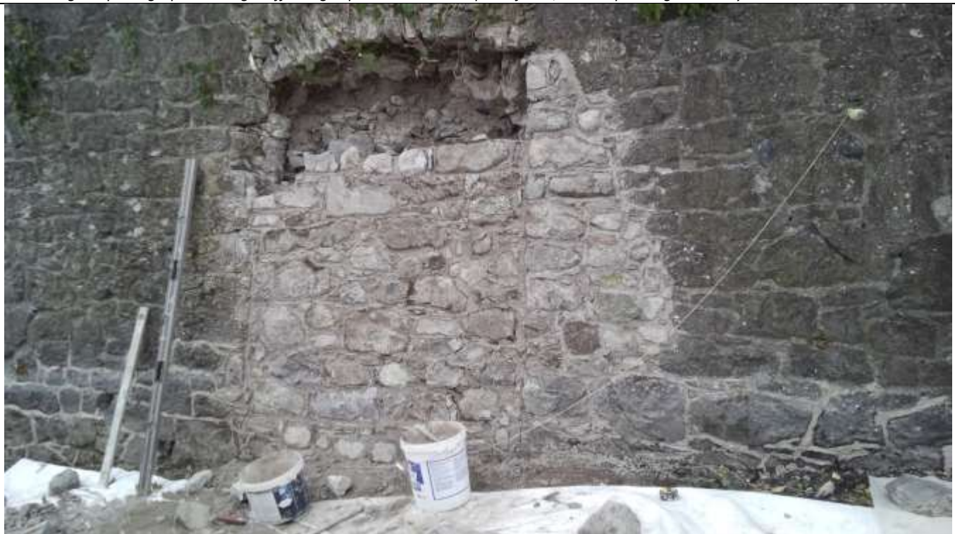
xiv. Progress photo showing reinstatement of stone rubble infill within earlier opening – October 2019
