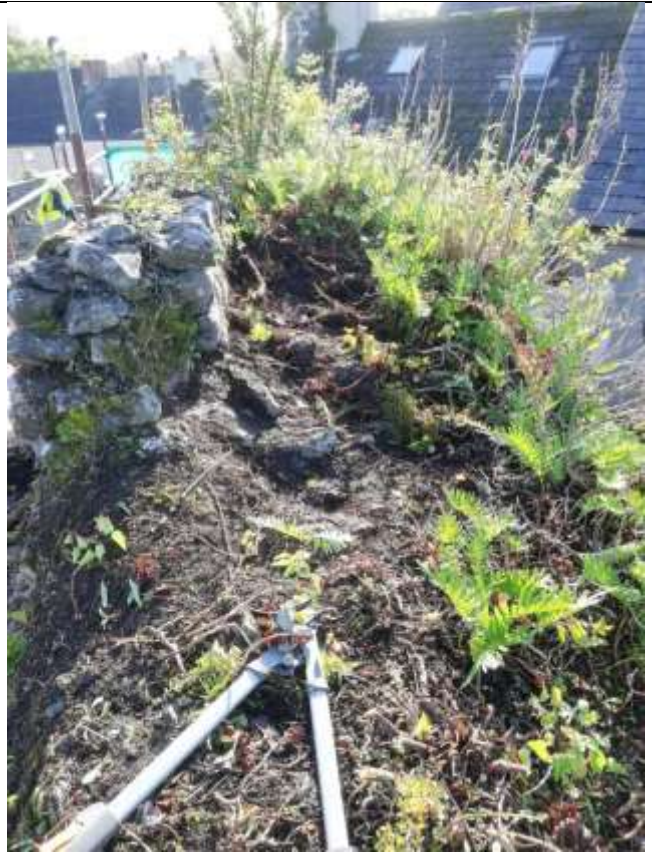
x. Significant levels of soil build-up were found once vegetation was removed from the top of the wall – progress photo October 2019
