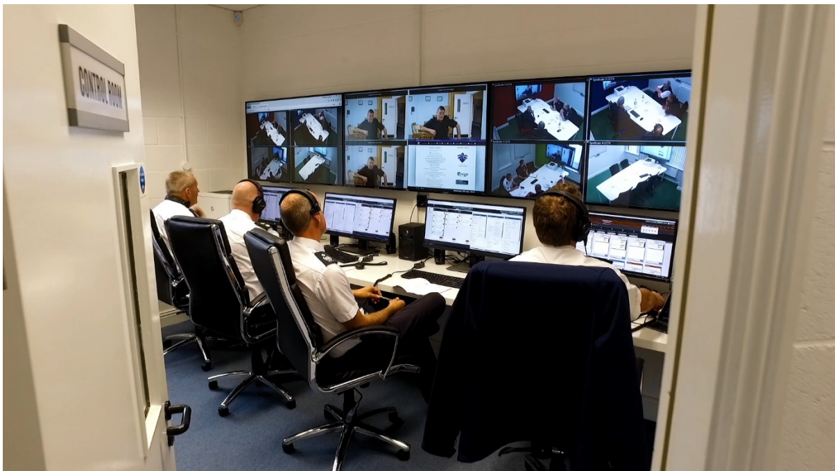
View of the HYDRA Suite Control Room
