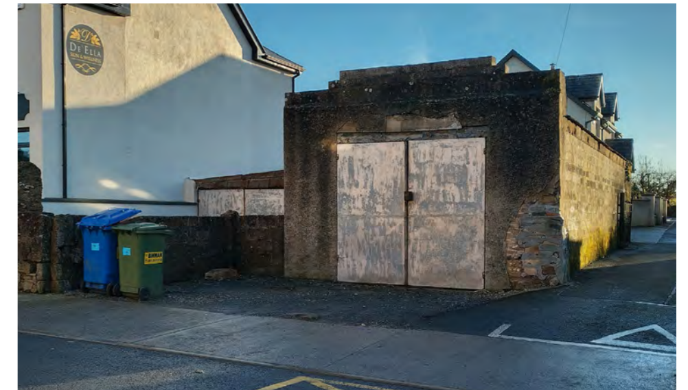
Vacant/ Derelict structure on Cork Road (2)
