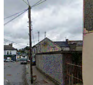
Timber utility pole
