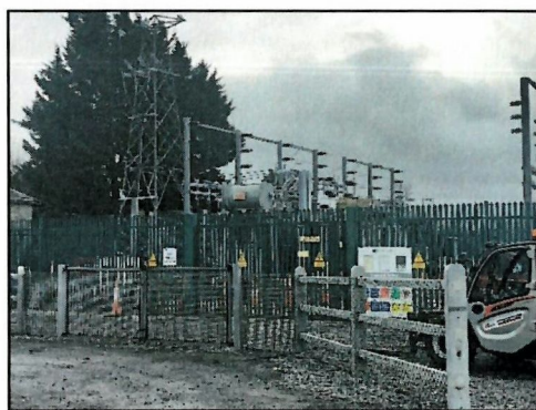
Plate 2-6 Existing Ardfinnan substation.
