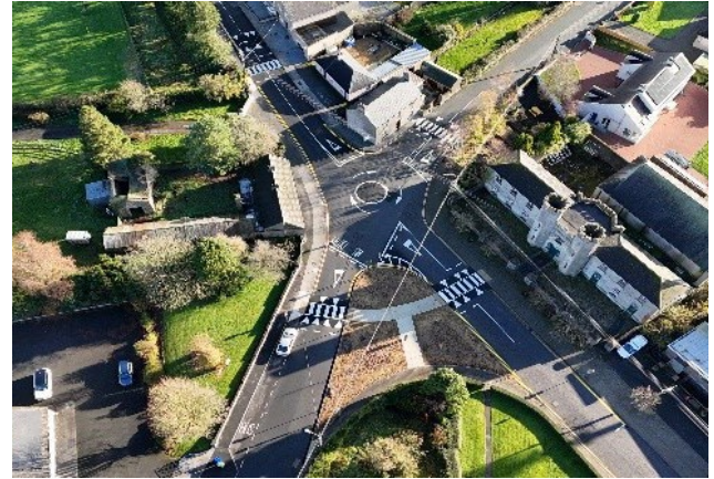
Improvement works at Corville Road, Roscrea, which includes installation of pedestrian crossings, associated ramps, landscaping and new footpaths.
