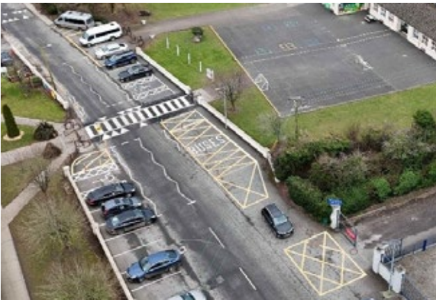
Pedestrian Safety Works at Borrisoleigh Primary Schools. Installation of 2-speed ramps, along with a Zebra pedestrian crossing, joining the two schools. The works also include pencil bollards, designated disabled parking bays and bus bays, and the refreshing of line markings surrounding the school.
