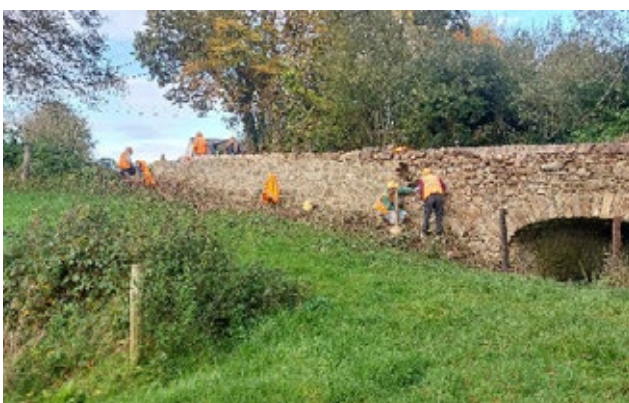
Repair work and building of stone wall on Deepark Bridge and Culvert on the R499 road from Dolla to the Silvermines
