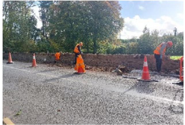
Repair work and building of stone wall on Deepark Bridge and Culvert on the R499 road from Dolla to the Silvermines
