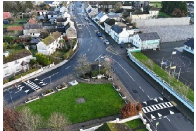
Improvement works at Templetoohy Village, to include 3 raised pedestrian crossings with associated signage and line marking, widened footpath, new bollards, new barriers & signs.
